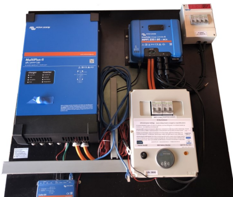
Off-grid System Equipment Board
