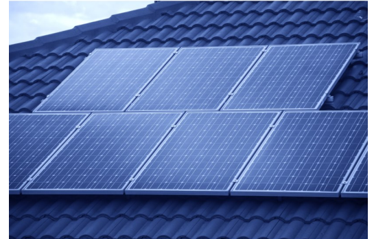
3.2KW Trina Solar Panels
