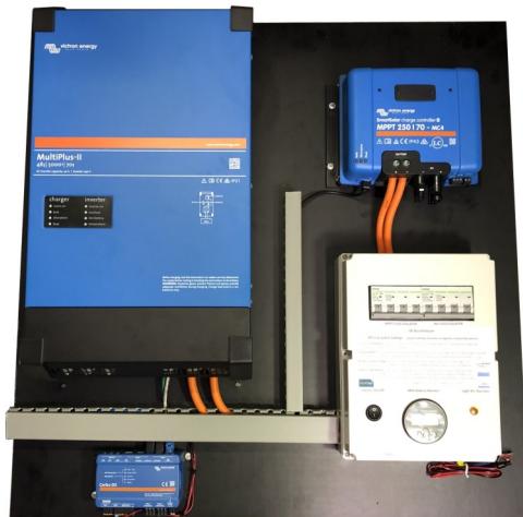
Off-grid System Equipment Board
