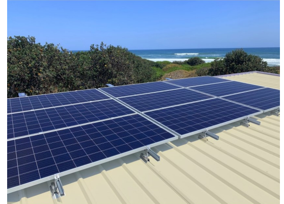
4.0KW Trina Solar Panels
